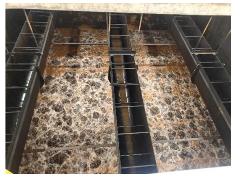
(b) Backwash air wash and filter boils
