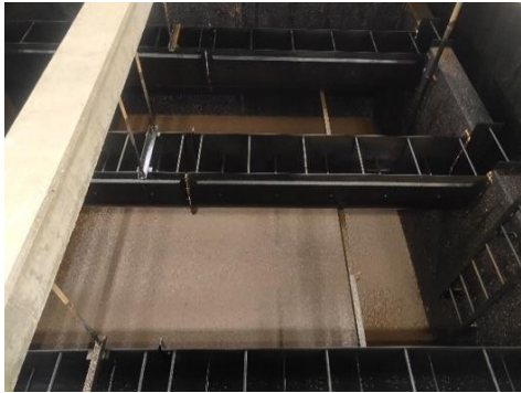
(a) The surface of the water filter medium before backwash
